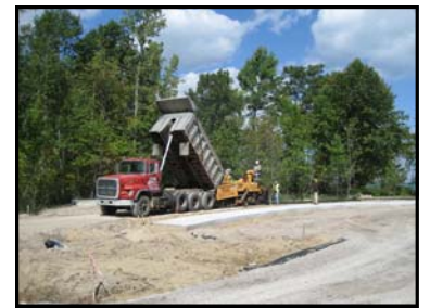
Workers install sidewalks during the construction of Fort Gratiot Park in Summer 2006
